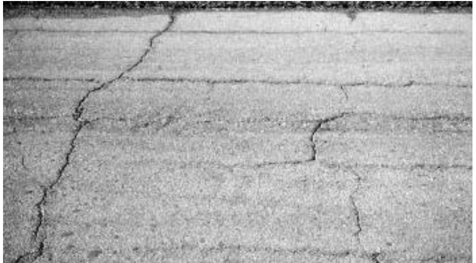
▼ Block cracking with open cracks.
