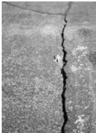
▲ Open crack – 1/2" or more in width.
