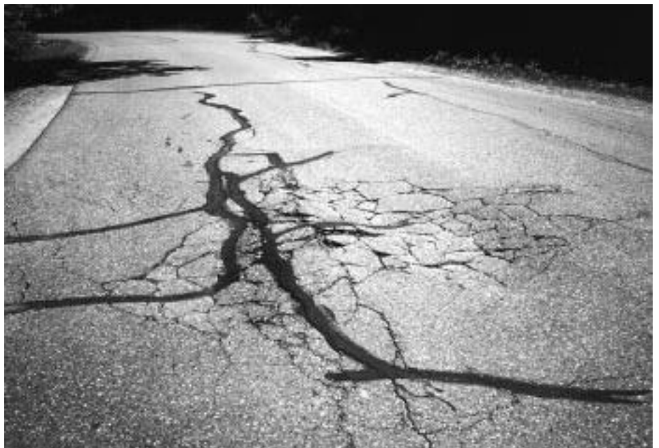
► Frost heave damage from spring break-up.
