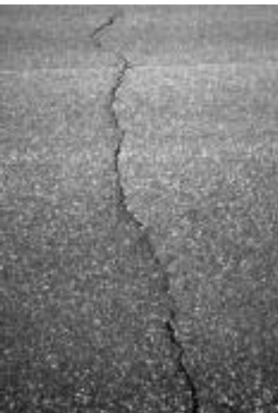
▲ Tight cracks less than 1/4" in width.
