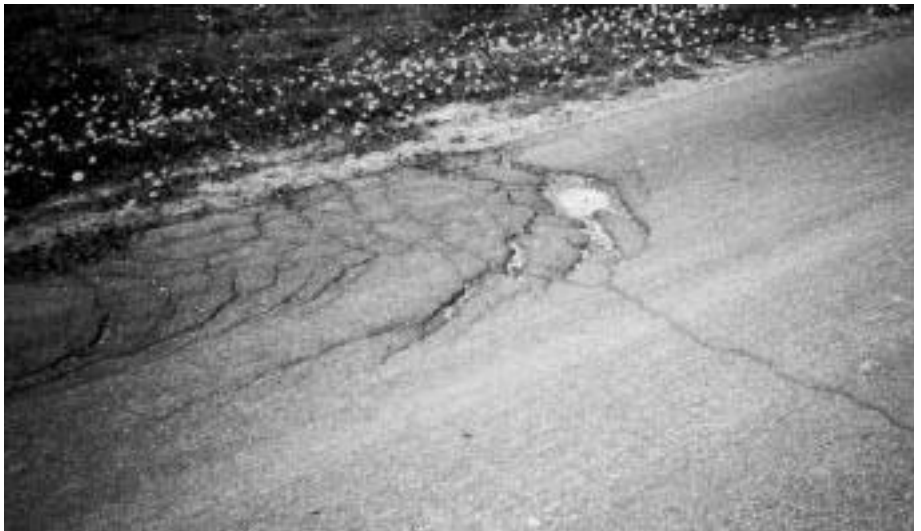
► Crescent-shaped cracks characteristic of slippage.
