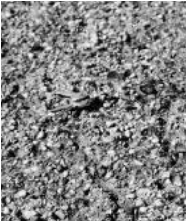
Severe raveling with ▼ extreme loss of aggregate.
