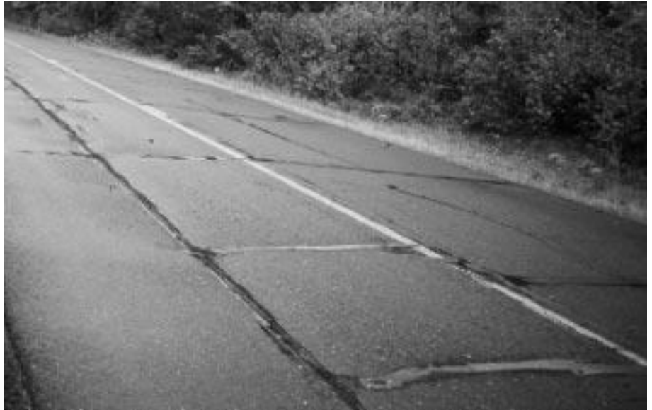
► Concrete joints reflected through bituminous overlay.
