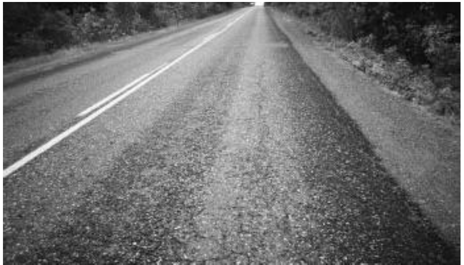
► Moderate to severe raveling in wheel paths.
