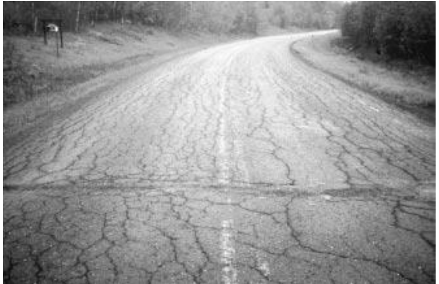
▶ Extensive alligator cracking. Pulverize and rebuild.
