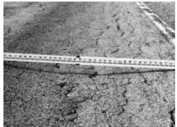
▲ Severe rutting. Strengthen base and reconstruct.
