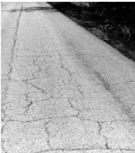
▲ Extensive block cracking in an irregular pattern.
